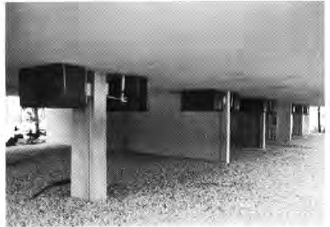
Figure 4.49. Elevated Condenser Units
